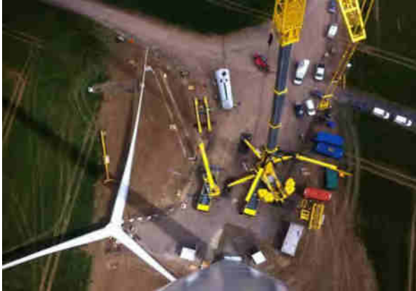
Hardstand for Assist Crane q2 (on slopes)Hardstand for Assist Crane q2 (on slopes)
