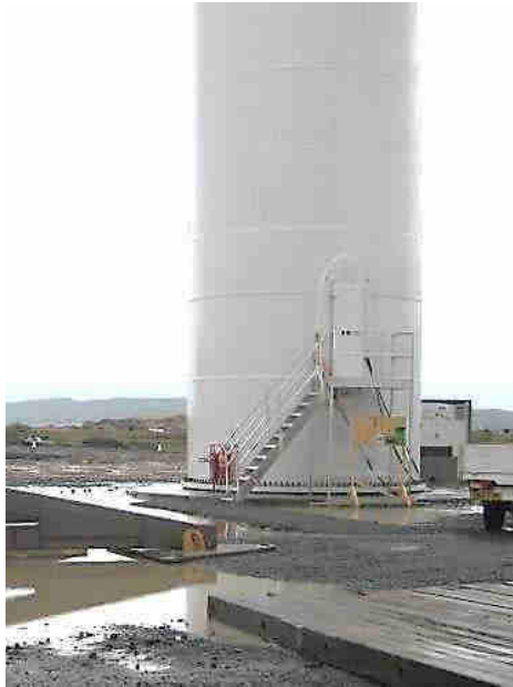
Figure 5: Example of not well-maintained service access to WTG.
