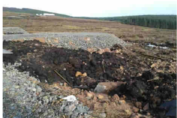
Figure 31: Example of an unacceptable/unprepared area between blade fingers.
