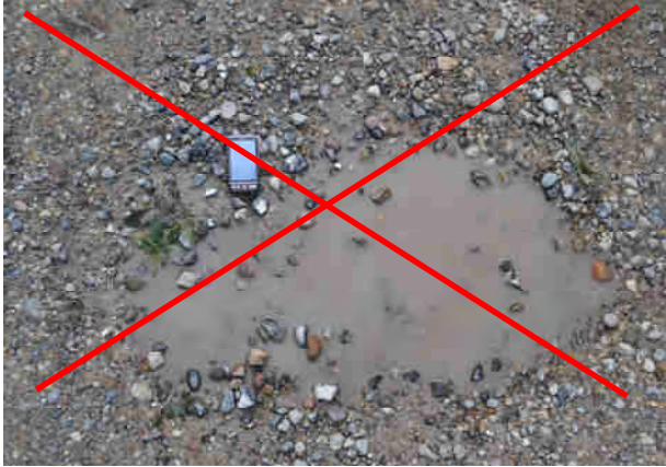
Figure 8: A well maintained Site Road shall not have pot-holes deeper than 30mm and/or a distribution/collection of pot holes that at the reasonable discretion of the Contractor cause unsuitable or unsafe driving conditions.
